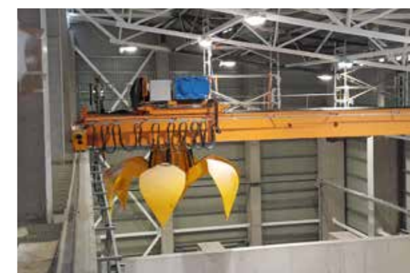
Automatic grab crane used in biomass energy plant (Customer „Axis“)
